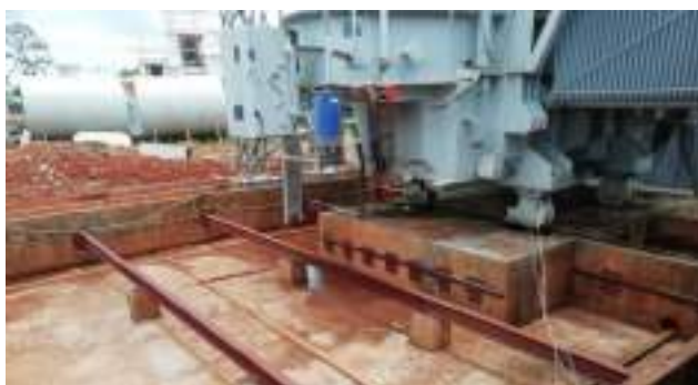
Plate 5.5: Transformer Oil Sump Pit at 220/132kV New Shillong
