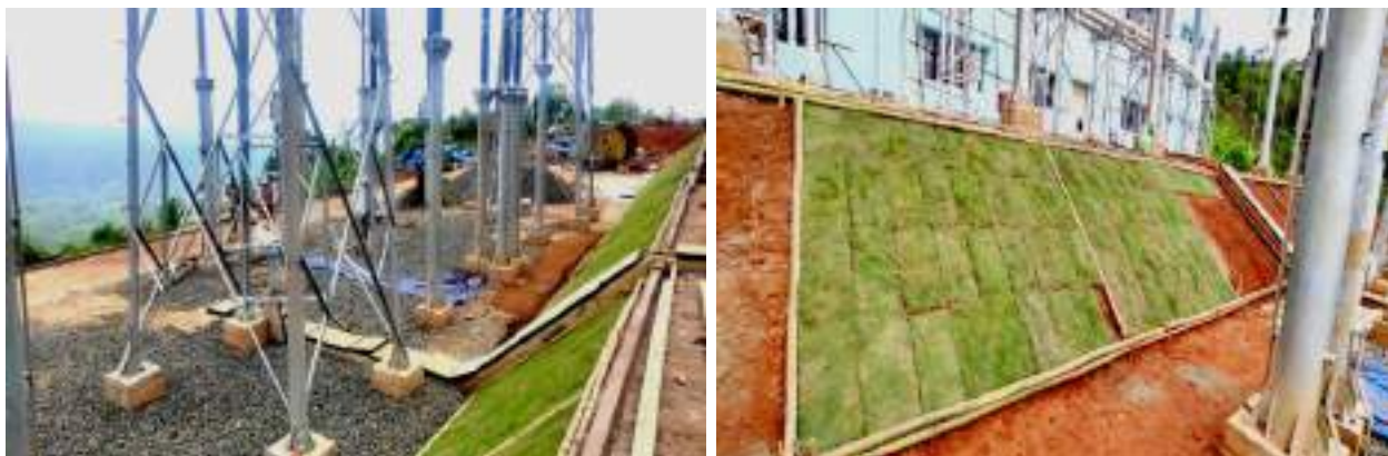
Plate 5.9: Grass with bamboo grids (Bio-engineering measures) for slope protection/ soil stabilization work under progress at 220/132/33 kV GIS Substation New Shillong
