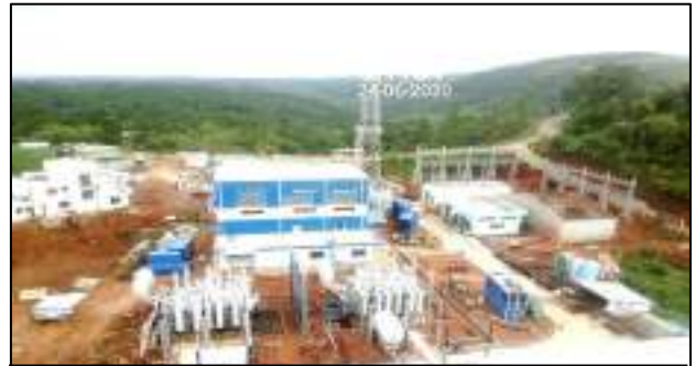
Plate-5.14 Activities confined within the substation boundary only
