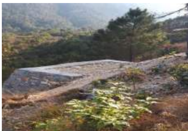
Plate- 5.10 Retaining Wall at 200 kV New Shillong Section at tower loc AP 76
